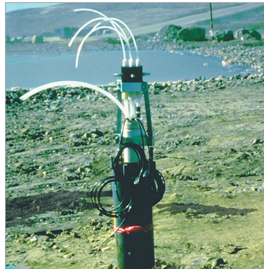
Landfill site over fractured granite, monitored with five Waterloo Systems. Each System comprised of dedicated Double Valve Pumps and Pressure Transducers in 4-6 intervals to depths of 84 m (275 ft). The Multi-Purge Manifold allowed the monitoring of 21 zones to be completed in less than 2 days.
