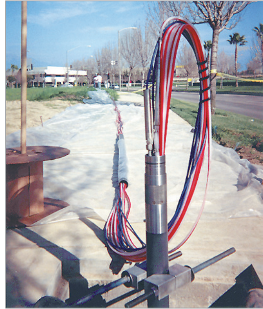
Contaminant investigation at a U.S. Air Force Base. Waterloo Systems installed to 213 m (700 ft) in overburden using screened and cased wells. Up to 6 zones per hole with dedicated pumps and transducers.
